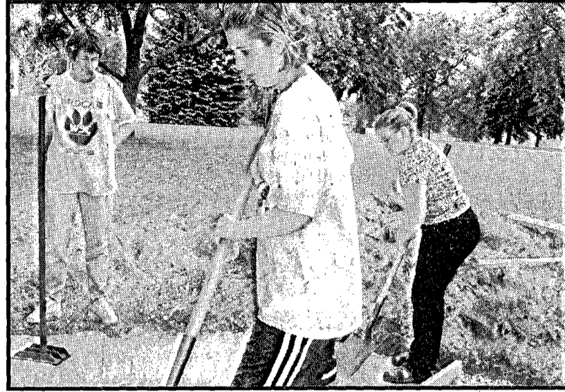
Left to right, Deb Daehnke takes a break from tamping while Lacey Webster and Amanda Hank shovel sand into the area around the fountain.
